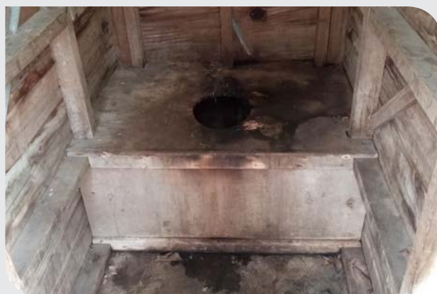
An example of a toilet in a health facility in Western Highlands Province.
